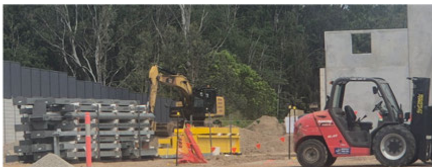
Skid off structural steel fabricated and painted removed from a sea container
