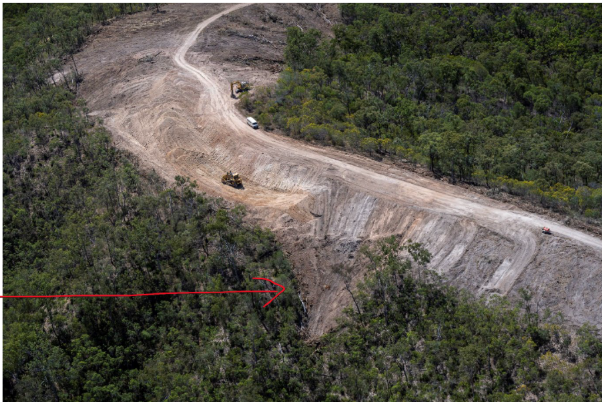
FIGURE 2 - BOULDER CREEK WIND FARM – NOTE UNCONTROLLED SEDIMENT / EROSION ALONG RIDGELINES
